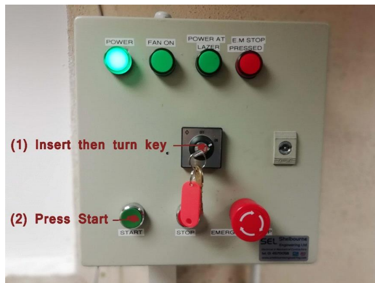
LEV Control Panel
